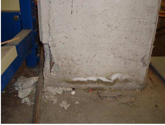
Fig. 6 Damage at the column base after the event on May 29 th
