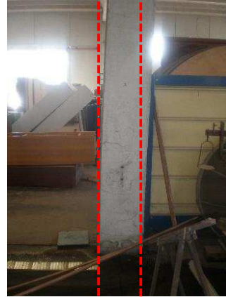
Fig. 7 Rotation of the columns around the global Y direction after the event on May 29 th
