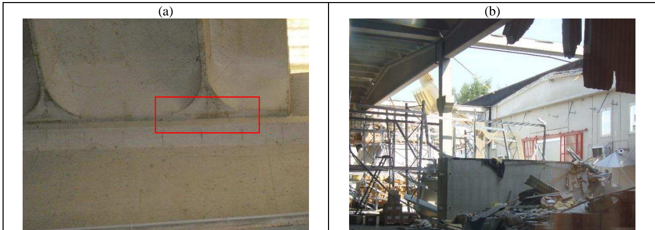
Fig. 9 Damage of the roof-to-beam connections after the event on May 29 th : (a) dislocations and (b) loss of support phenomena
