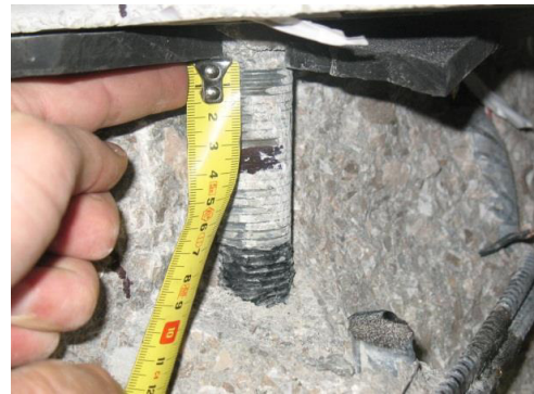
Figure 21. Measurement of the plastic hinge depth in the steel dowel after the monotonic test
