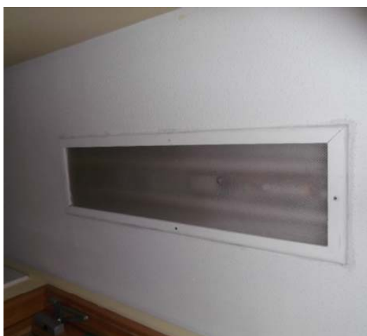
Figure 2: Exemplar undamaged light fitting
