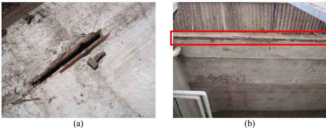
Figure 12. Collapse of vertical precast panel connection: (a) the anchor channel embedded in the panel and the failed hammer head element; (b) profile located in the beam which the hammer head elements are welded to.
