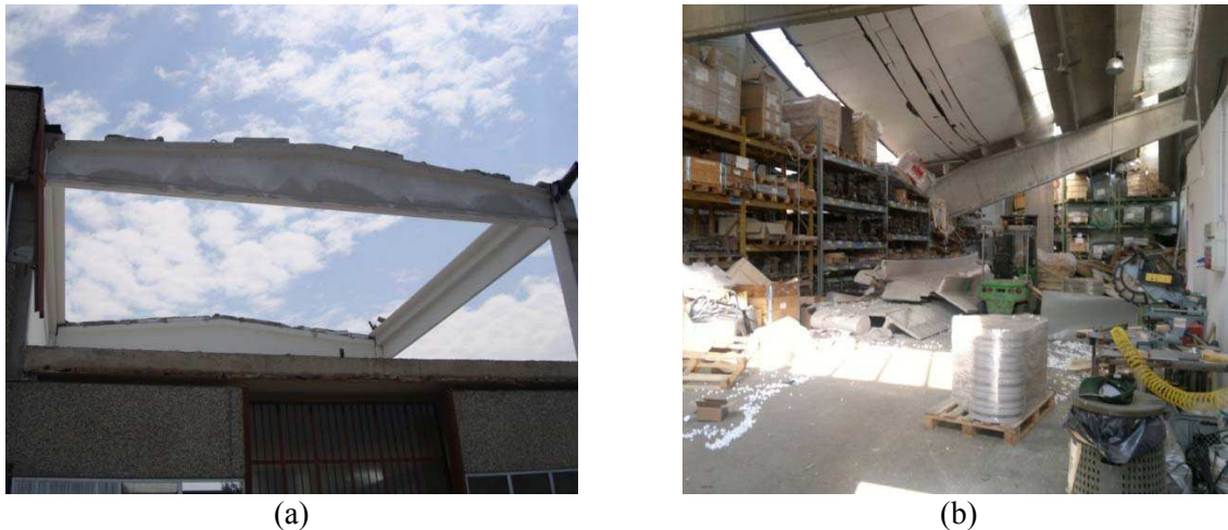
Figure 5. (a) Roof elements collapse due to the loss of support from main beam. (b) Loss of support of beam from column.
