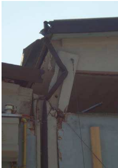
Figure 9. Shear collapse of column due to the interaction with infill masonry panel.
