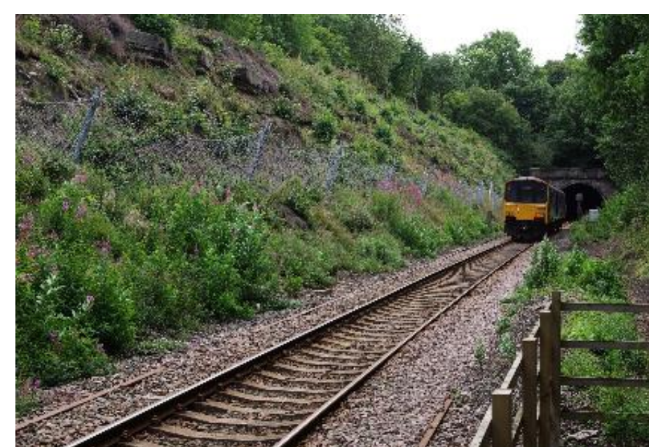
Fig. 4 A rockfall catch fence on a hillside next to a train line.
