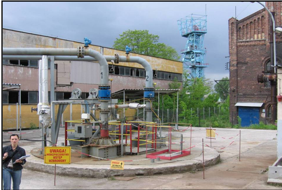
Figure 1. Katowice mine shaft (with dewatering pumps) in an urban environment in Poland (photo by © David Banks).
