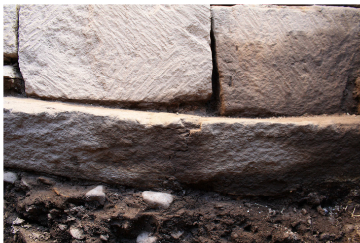
Fig 5 Detail of toolmarks on tower plinth 4707 (above), and lack of them on early structure 4711 (below)
