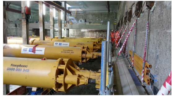
Figure 2: Inside the station main box with sensors installed in far corner.
