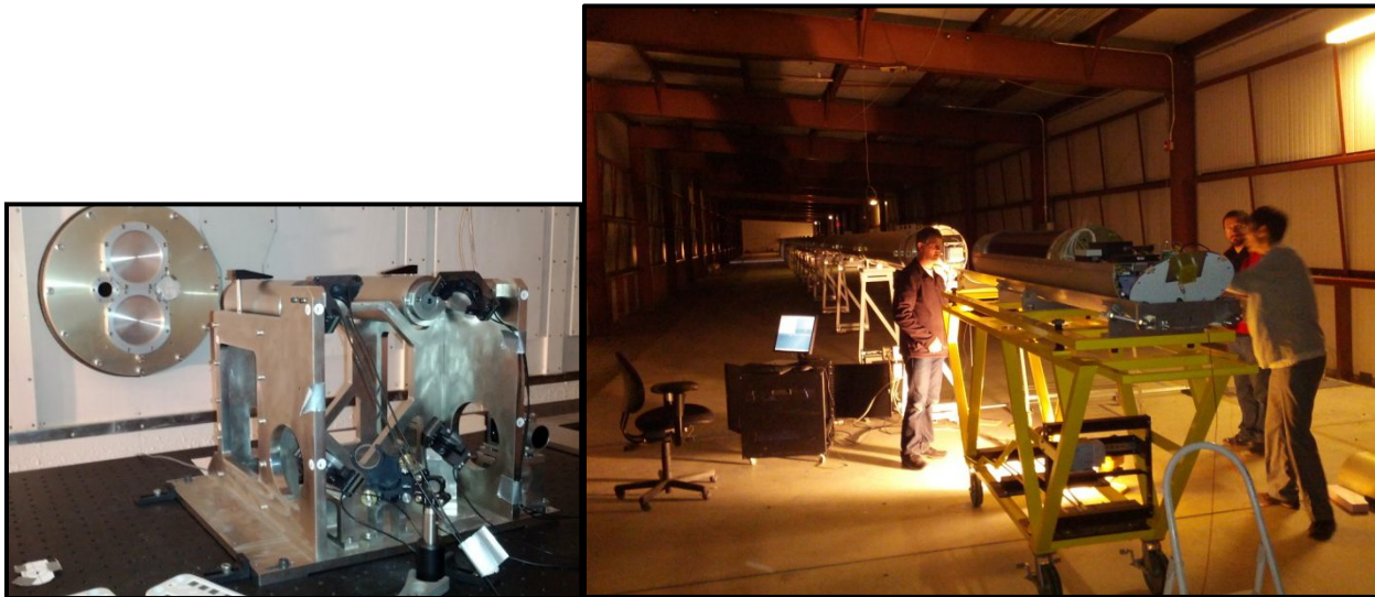
Figure 8: Successful installation of delay line pipe and trolley at MROI. On the left is shown the metrology launch table within the inner beam combining area, while on the right is an image from SAT work during the installation of trolley #1 into the 100m delay line pipe.
