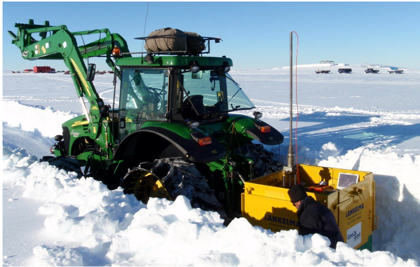
Figure 5.28: Overburden was sequentially removed by bulldozer to enable assessment of resistance variation under varying confining pressures.
