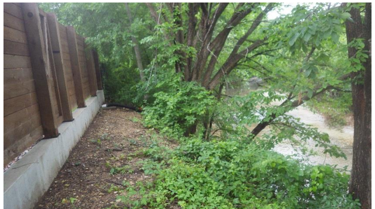
Photograph 24 – Private property retaining wall and fence with attached outfall, view to the east.
