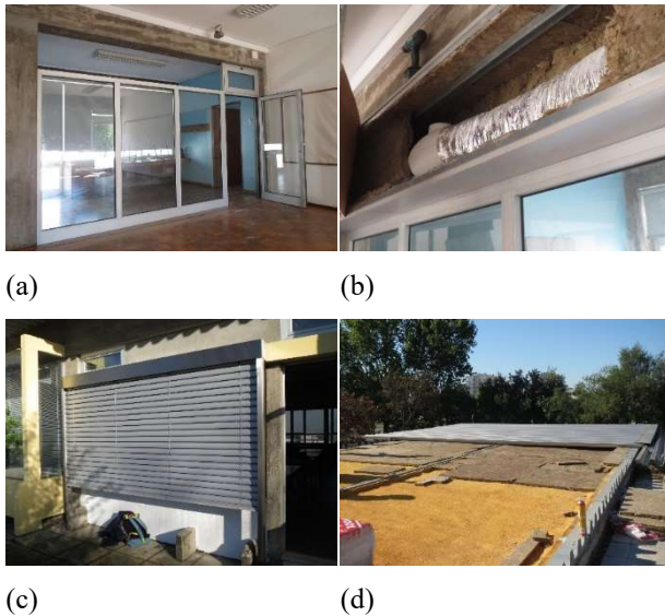
Fig. 2. Prototype interventions: (a) partition wall; (b) ventilation system; (c) exterior blinds; (d) roof insulation.
