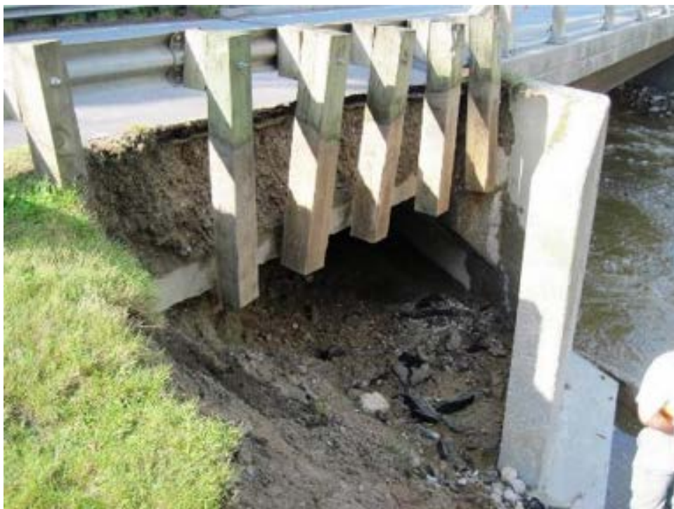
(b) Jamaica VT30-B40 Bridge: flanking behind the abutment undermining the approach slab
