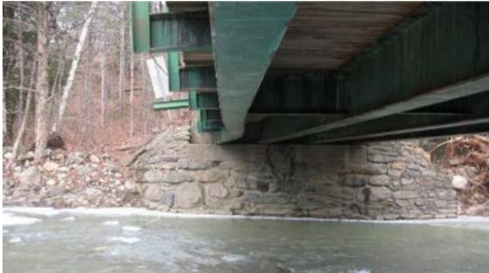
(b) Marlboro C3014-B23 Bridge: damage to the main beam of the bridge from debris impact
