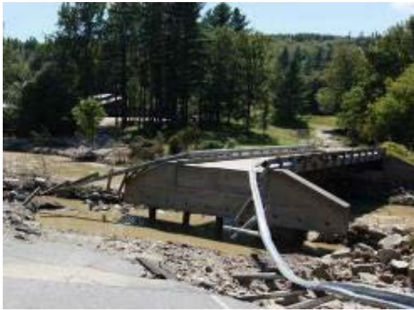
(a) Scour behind an abutment of a bridge in Ludlow, VT (source: Burlington Free Press)
