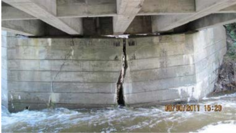
(a) Brownington C2001-B9 Bridge: fracture to the foundation, due to scour beneath the footing and settlement of substructure
