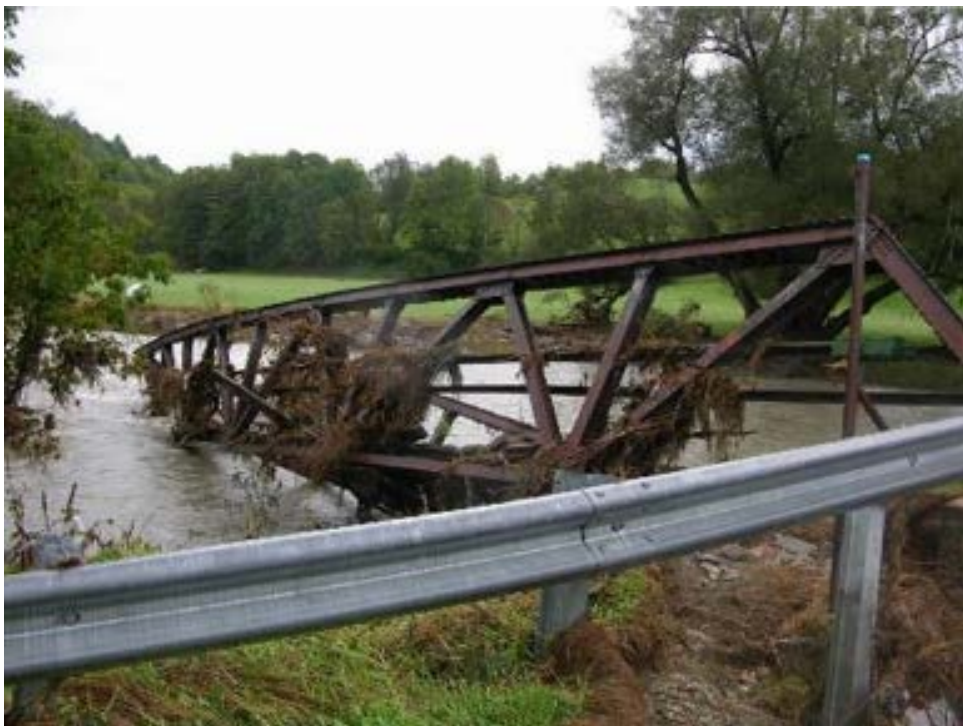
(b) Moretown C3024-41 Bridge: collapse of the steel truss bridge from the apparent loss of one of the bridge foundations
