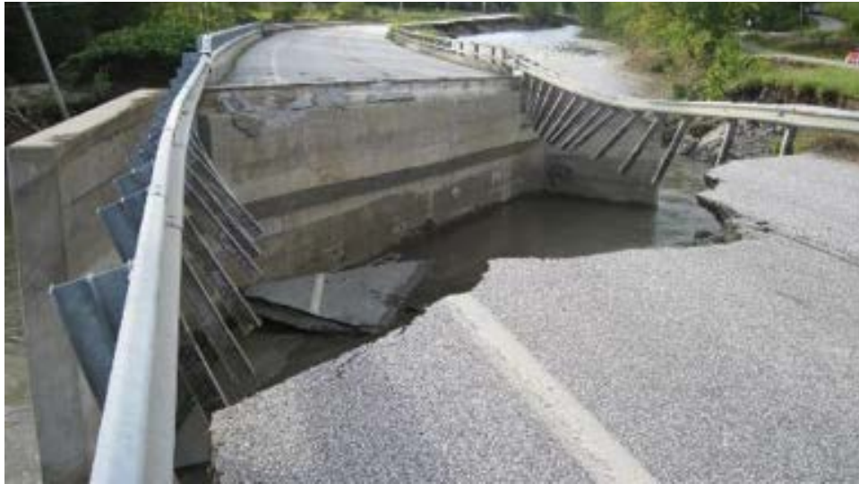
(a) Braintree VT112A-B6 Bridge: erosion behind the wing-walled abutment, with complete loss of the bridge approach
