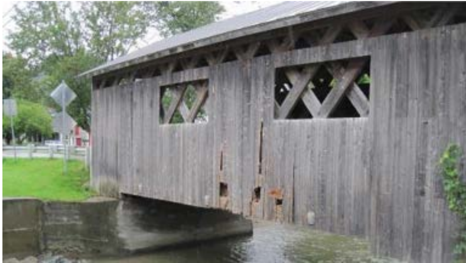
(a) Montgomery C2001-B5 Bridge: damage to the sideboards of a covered bridge
