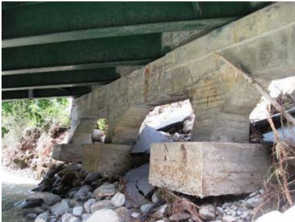
(b) Jamaica VT30-B78 Bridge: flanking behind the wingwall abutment, with scour beneath the bridge foundation, with no apparent damage to the concrete foundation, and no major settlements to the foundation
