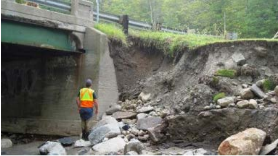
(a) Wardsboro VT100-B68 Bridge: flanking erosion behind the abutment, and minor scour to the footing
