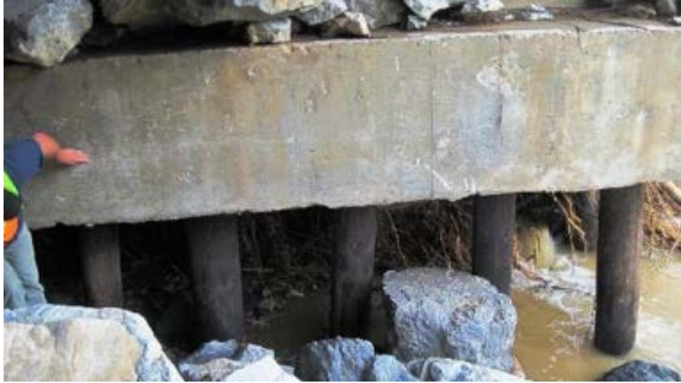
(a) Clarendon US7-B96 Bridge: scour beneath the foundation, exposing several feet of wooden piles
