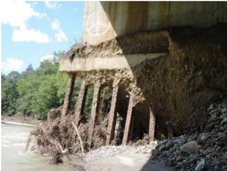
(b) Dummerston VT30-B9 Bridge: scour beneath the concrete spread footing, with settlement resulting in the cracking of the foundation.
