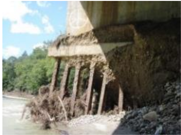
(b) Abutment scour in Dummerston, VT (Source: VAOT)
