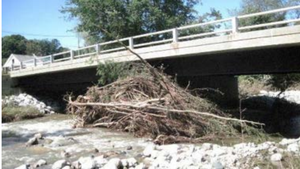
(a) Wallingford VT140-B10 Bridge: debris buildup on a pier, reducing the flow area
