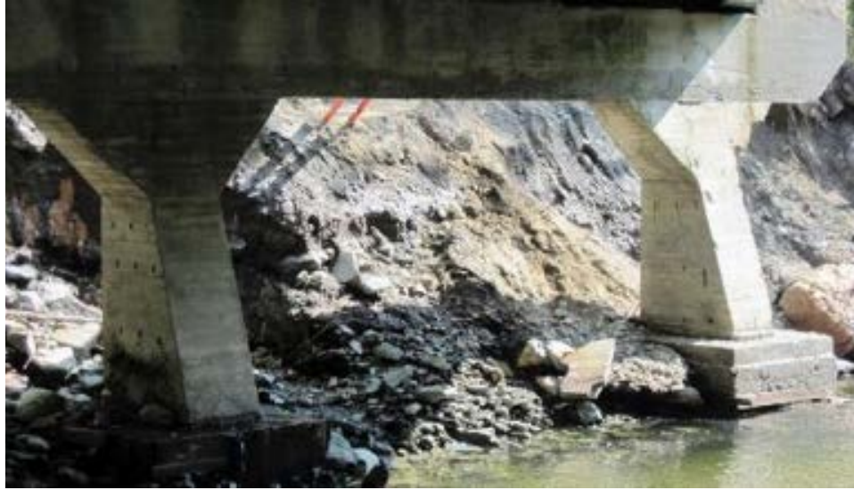
(a) Halifax C2001-B17 Bridge: loss of original riprap and backfill, resulting in the free standing abutments and scour to beneath the footing of the spread footing base
