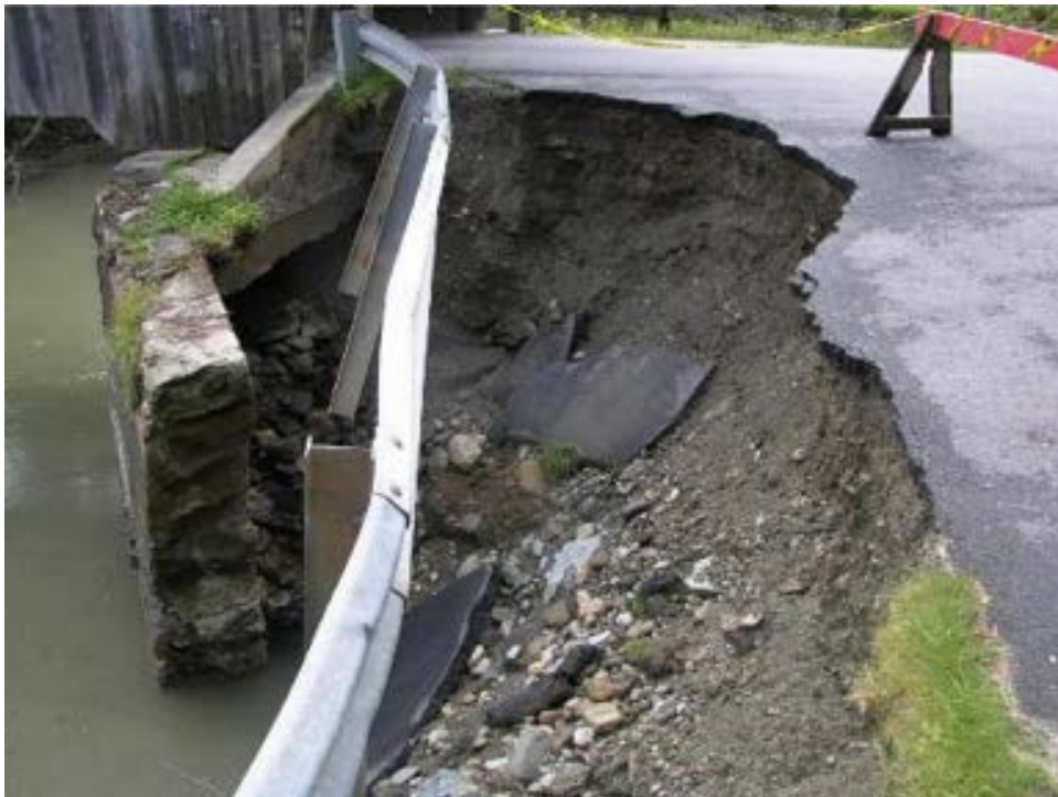
(b) Warren FAS188-B6 Bridge: Channel erosion and flanking behind the wingwall, with scour hole at the toe
