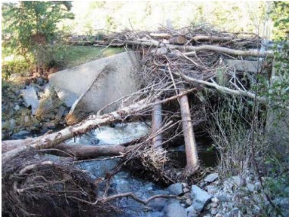
(b) Wilmington VT100-B53 Bridge: obstructions at a small single span resulting in blockage and overtopping
