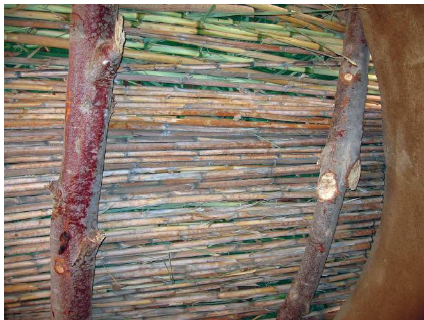
Figure 15 Roof construction with wooden beams supporting reeds (in turn supporting mud), seen from below.
