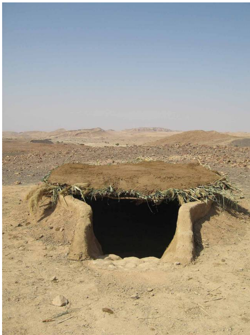
Figure 16 The finished structure in its surroundings (looking north-west). The mud-covered roof is clearly visible.
