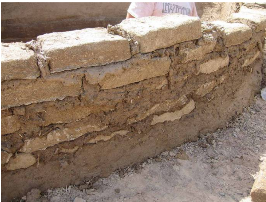
Figure 13 Mudbrick wall, bound with mortar and in the process of being covered with mud plaster.
