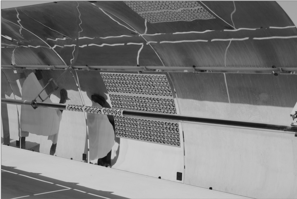
Figure 4.32 - Saudi Arabia parabolic trough set up
