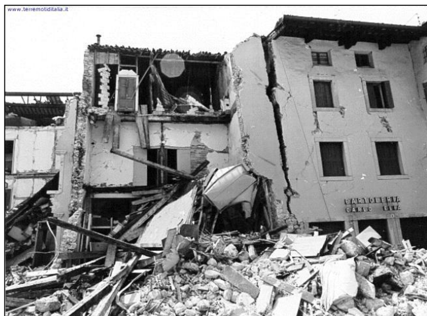
Figure 3.5: Friuli, impact of earthquake on a local bar
