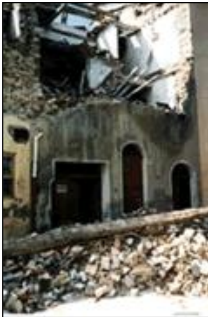
Figure 3.7: Destroyed home after Umbria-Marche earthquake
