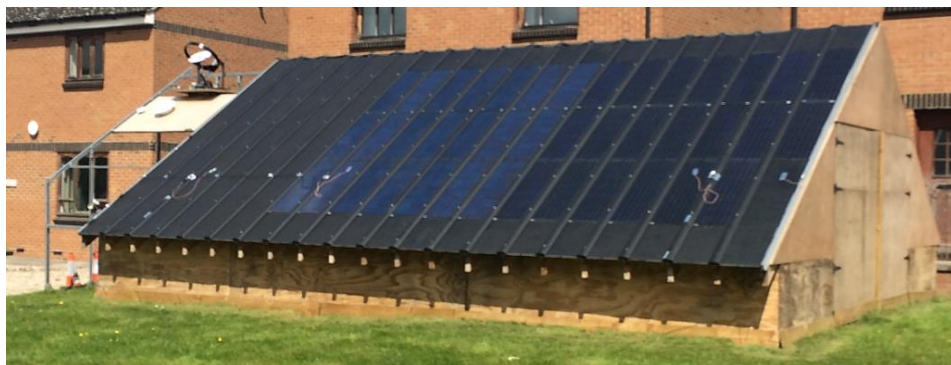
Figure 2: Solar hybrid PV/T test installation view
