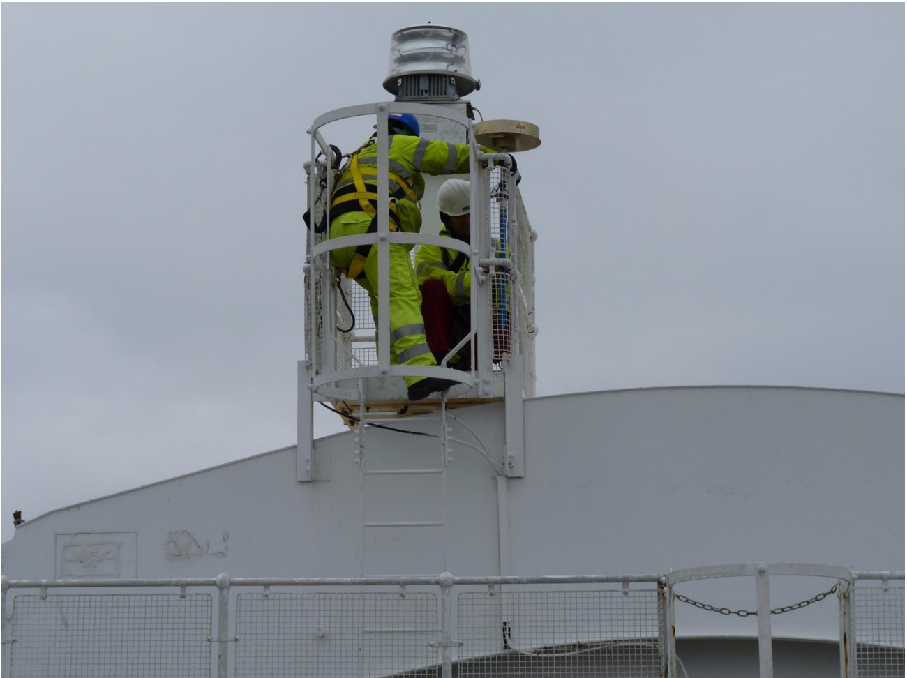
Figure 4. The GNSS antennas located at survey point T2 on the bridge. The illustration shows the GNSS antenna being installed
