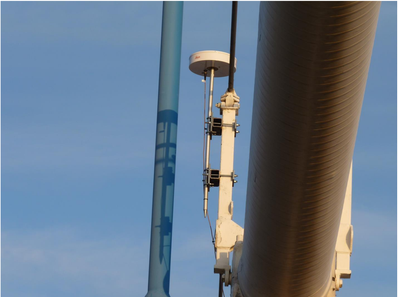
Figure 5. GNSS choke ring antenna located on the suspension cable.
