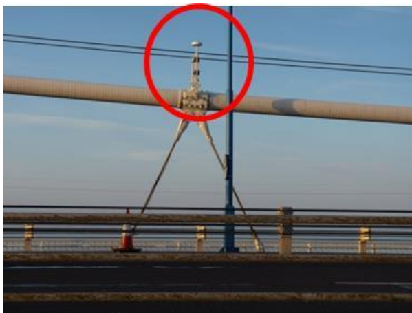
Figure 8, A GNSS antenna located on the Severn Suspension Bridge's suspension cable, Location C.
