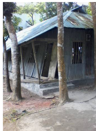
Damage in the Cyclone Mahasen in 2013
