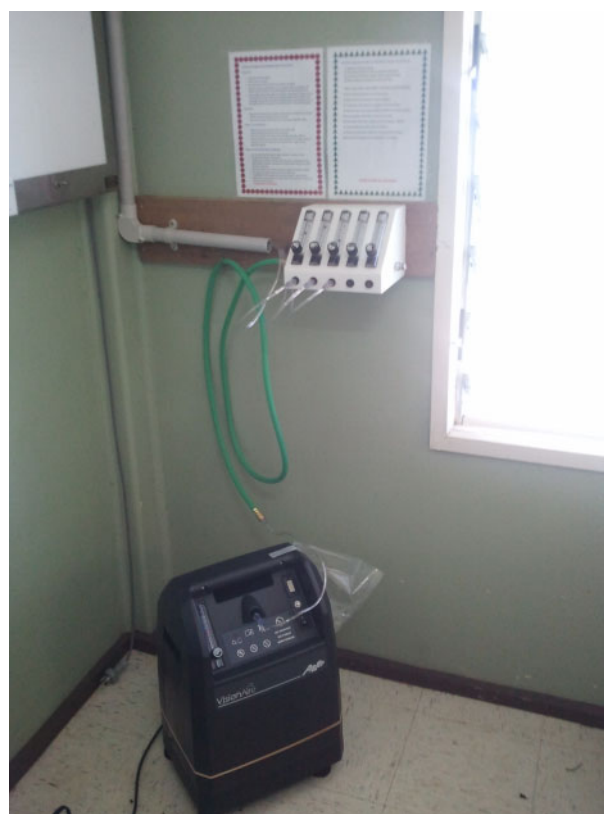
Figure 1 The oxygen concentrator after installation. Note the laminated instructions on the wall, the flow meter connected to the concentrator oxygen outlet, and the oxygen tubing running from each flow meter outlet through conduit to reach each bed-side
