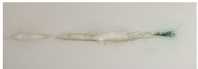
Fig. 5: Damage in the back sealing surface behind the busbar; tear, blister, humidity ingress are visible.
