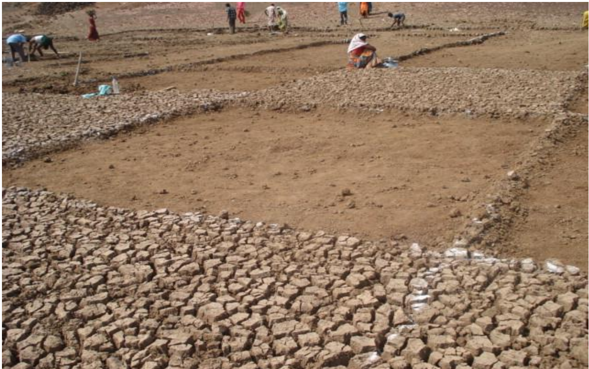
Photo 7-2: NREGA Pond Deepening Worksite – 2012 12 ft x 12 ft * 1 ft deep plots marked as daily work for a pair of workers
