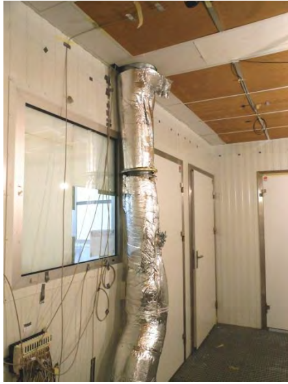
Figure 5.5 – Ventilation supply duct
