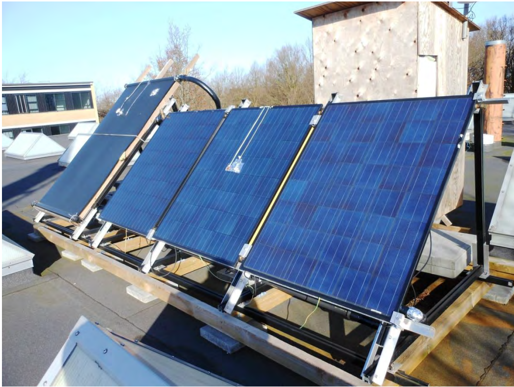
Figure 5.15 – Front view of the solar collectors
