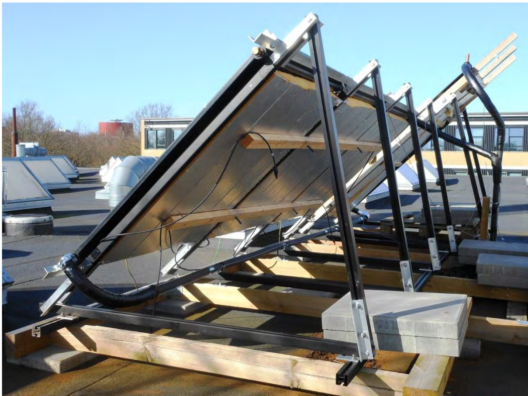
Figure 5.16 – Rear view of the solar collectors
