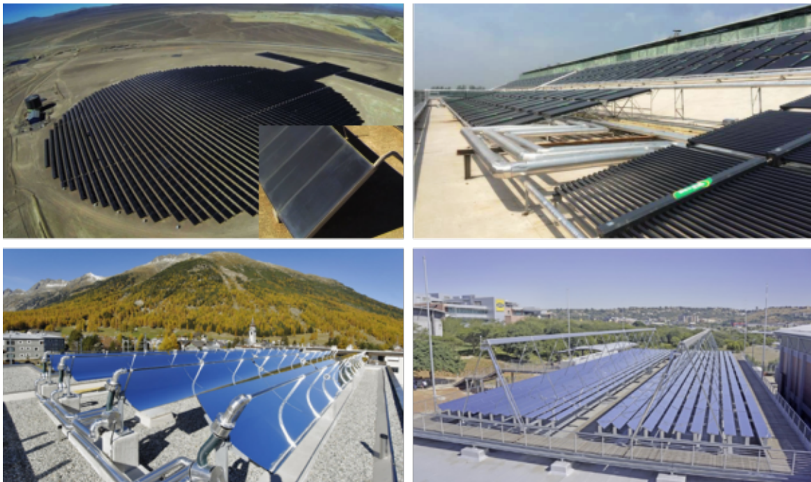
Fig. 1.7 Different examples of SHIP plants: A flat plate collector plant for mining (Chile), an evacuated tube collector plant for the textile industry (China), parabolic trough collectors for milk processing (Switzerland) and LFCs for cooling (South Africa).
