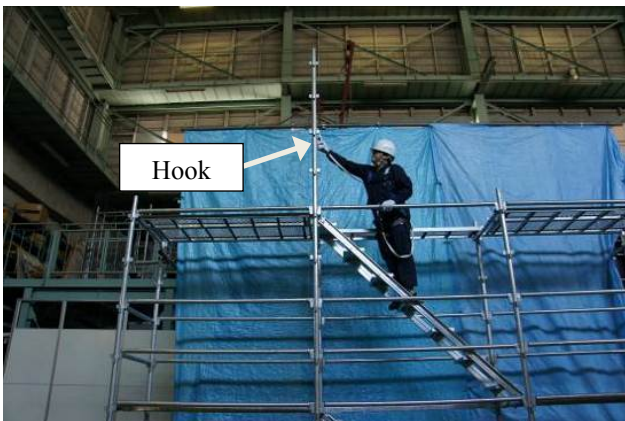
Figure 9: The worker who tried climbing the stairs to the next platform.
