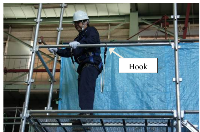
Figure 12: The worker who tried setting other members with hanging the hook of the harness to the guardrail.
