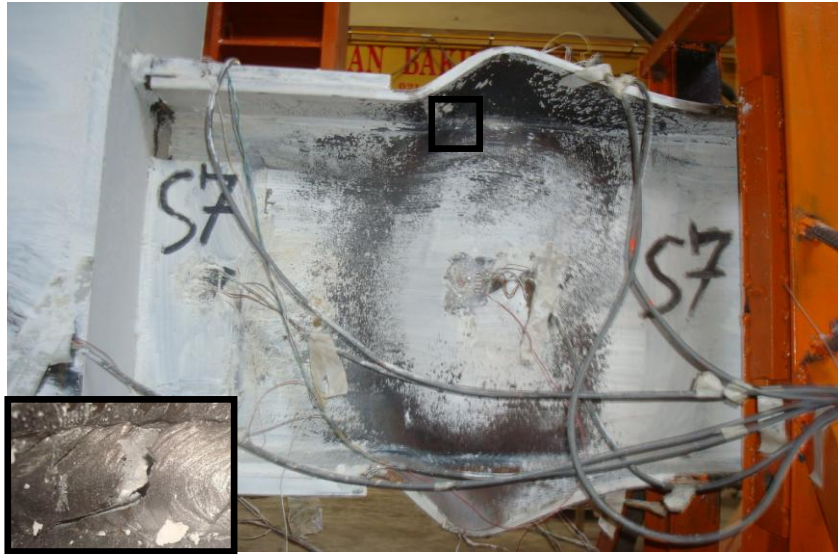
Figure 5: Fracture at the groove weld joining the beam web to the beam flange in the BD
