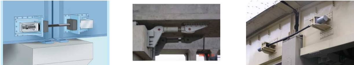
Figure 3 Schematic of expansion joint with various restrainers configurations: (a) through the hinge – Configuration I, (b) through the pier – Configuration II, (c) through hinge with shear key – Configuration III
