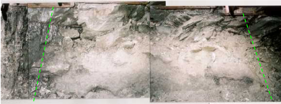
Fig. 9 Old roadway observed in Jobu Hidari No. 5 SD. Old roadway was closed by the deflected and sagged roof. Rocks below the deflected roof were softened.
