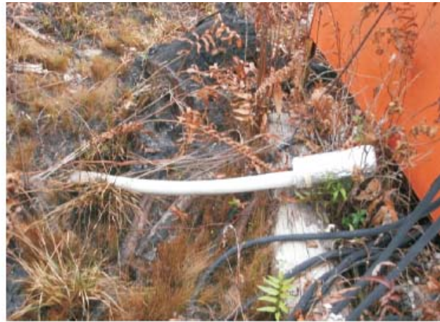
Fig 47. All of cable for gasses measurement was burned (Japanese tower, 05.10.09)
