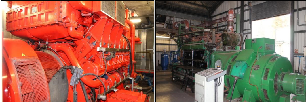
Picture 2-B: Paxman (left) and Blackstones diesel generator (right)
