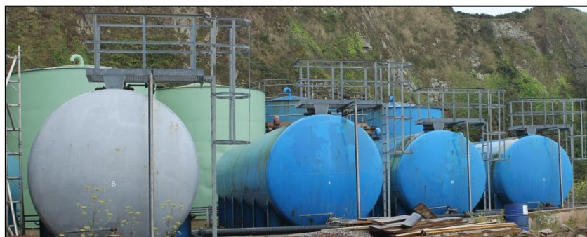
Picture 2-A: Diesel and kerosene storage tanks
