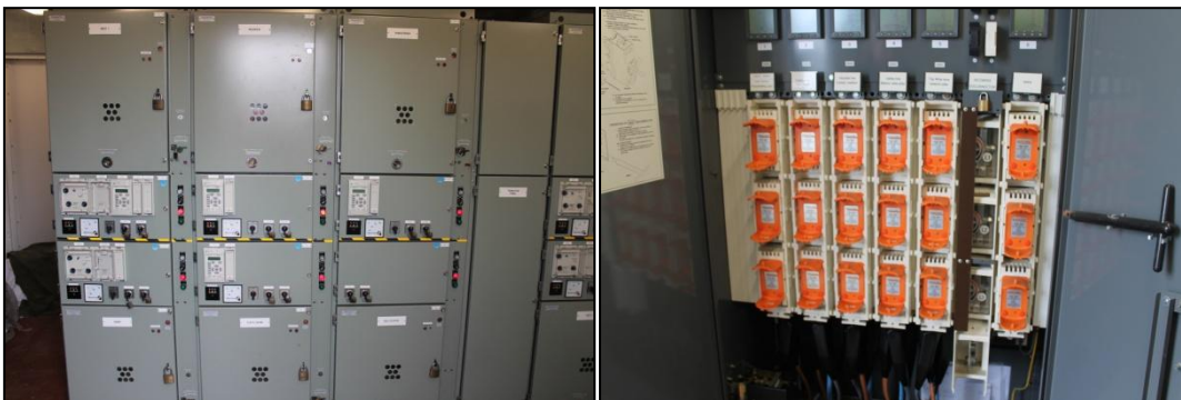
Picture 2-D: Switchgear and main switches of a modern substation
