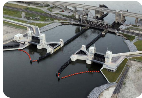
Image 62. Porte anti-inondation Seabrook
