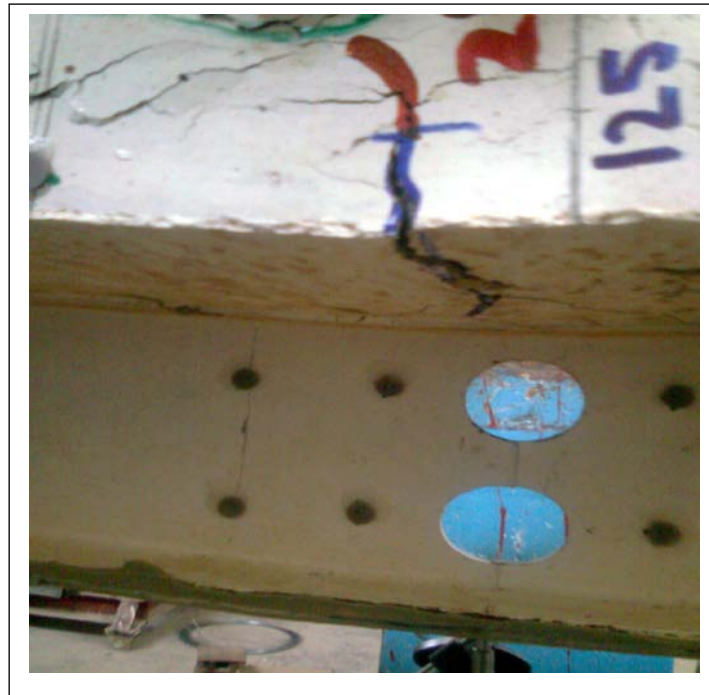
Figure 5: Beam CBSO2 at failure
