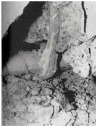
Figure 4: failure in stirrups at the bent zone of L05-1 (Bentz et al. 2010)
