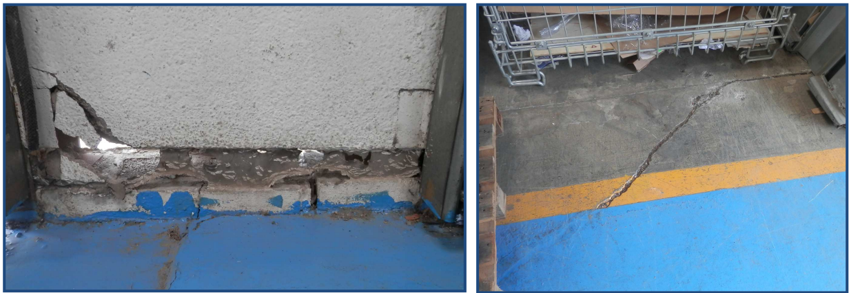
Picture 3.2.2a – At left we can see the settlement of the slab in the encounter with a facade wall. At right, the cracking of the slab when not being able to withstand the deformation.
