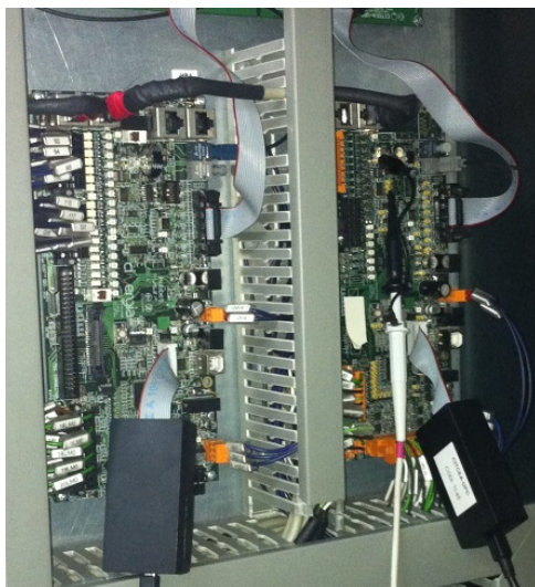
Figura I.6: Plaques de control
