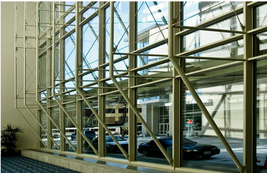
Figure 2.1. Three-dimensional tension truss system; Walter E. Washington Convention Center, Washington D.C., U.S.A.
