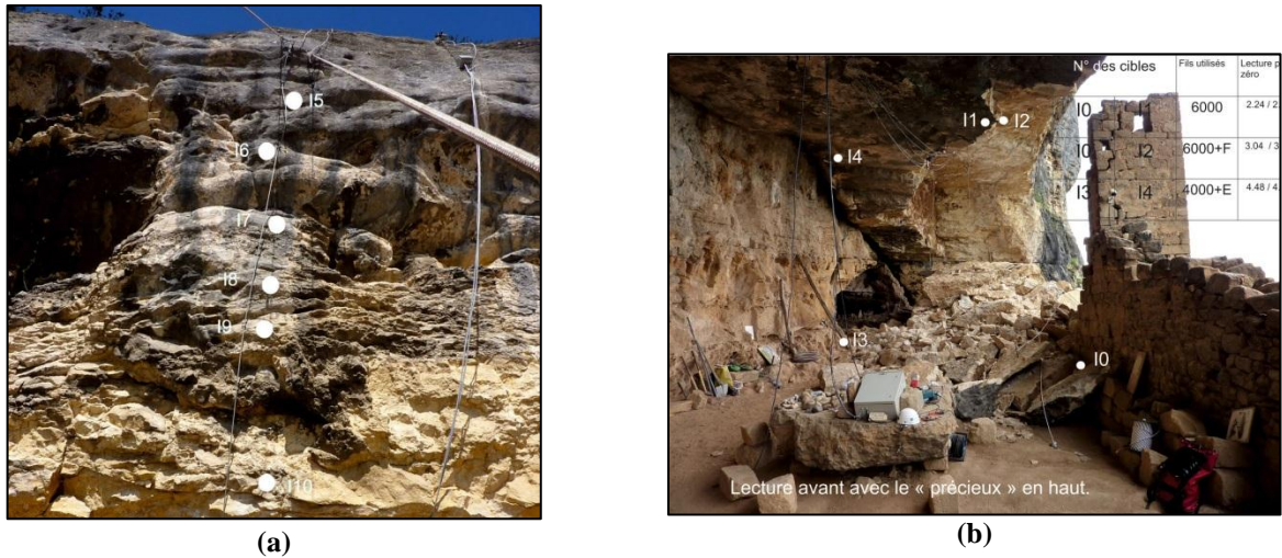
Figure 3-21. Convergence Measurements; a) Superficial spots located on one vertical line at top of the cavern; b) Within the cavern
