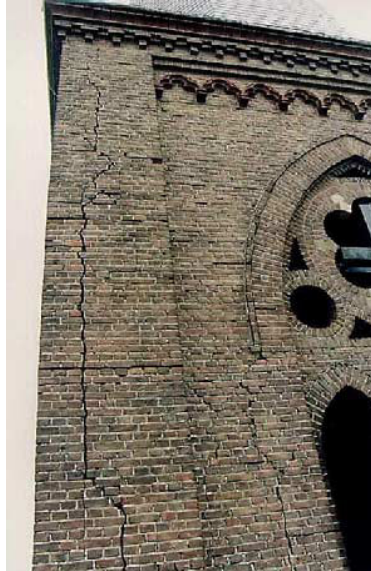
Figure 13 Church tower in Noordwijk, with both vertical and horizontal cracks (van Hees et al, 2003).
