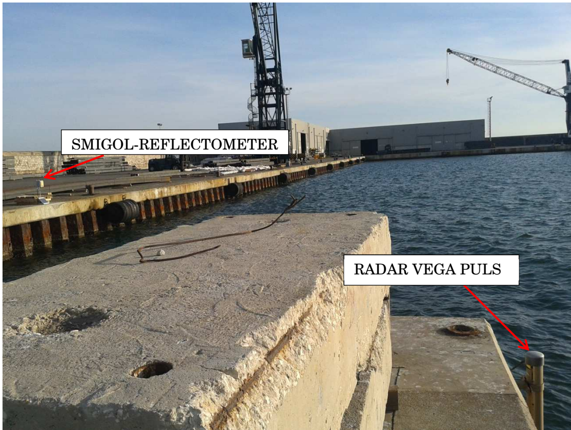
Figure 5.2: SMIGOL Reflectometer and RADAR VEGA PULS [16].
