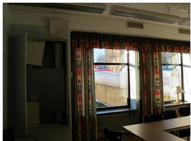
Figure 51: Room with his own supply air system 2
