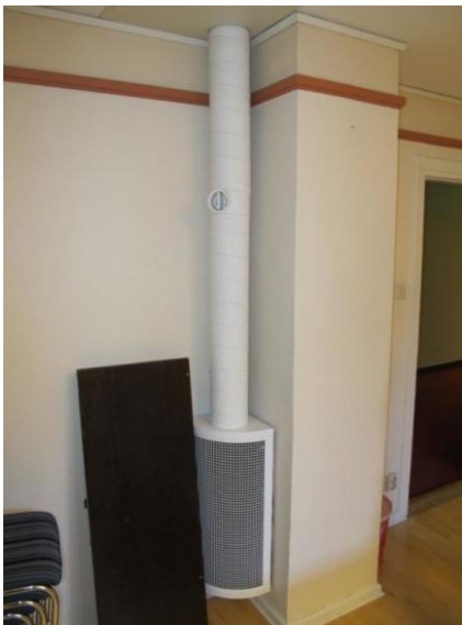
Figure 50: Room with his own supply air system 1
