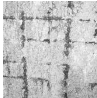
Fig. 6.1.6 Corrosion of the nets
