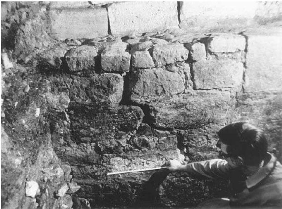
York Minster exploratory excavation 1967: The imposition in the fifteenth century of the 16 000 tons Central Tower on the eleventh-century foundations, intended for a much less heavy crossing, caused differential settlement which distorted and cracked the foundation masonry.
