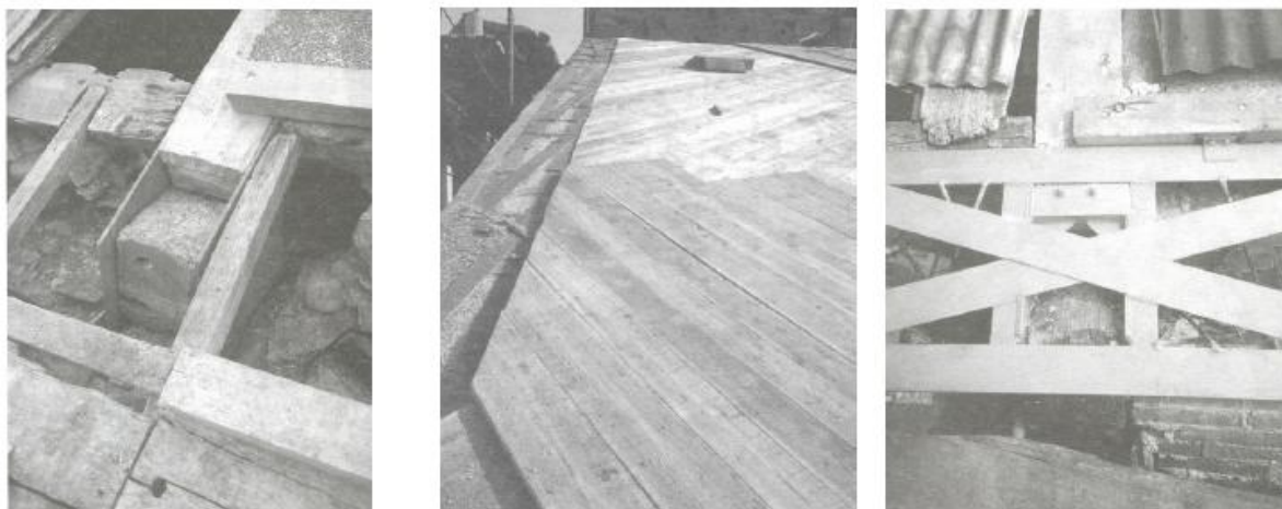
Figure 5.2.6.5 Steel ring beam: a) connection between the wood roof element and the walls; b,c) partial strengthening of the plywood panel diaphragm and its connection with the steel ring beams (Regione Marche 2000).
