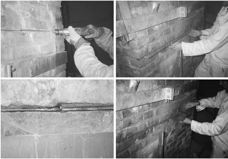
Figure 5.2.5.12 Phases of excavation, positioning, pinning and repointing of a damaged pillar (reinforcing rings were then removed)
