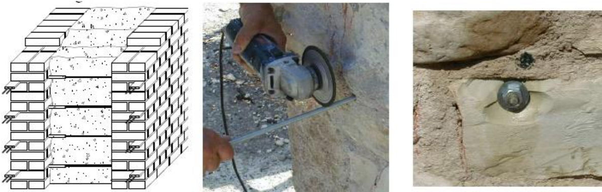
Figure 5.2.6.7 . Strengthening solution for pier walls: a) restoring of mortar joints and installation of steel bars, b) transversal bars bolted through washer.
