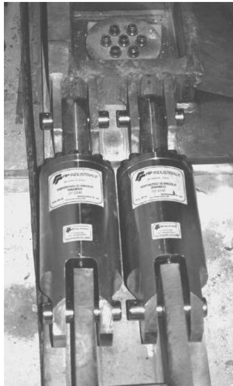
Figure 5.3.5.3 - A pair of 220 kN shock transmission units installed in the Basilica.
