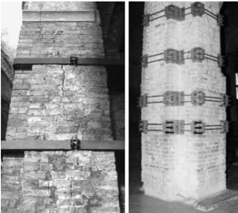
Figure 5.2.5.11 Church of S. Sofia in Padova: provisional measures on cracked pillars
