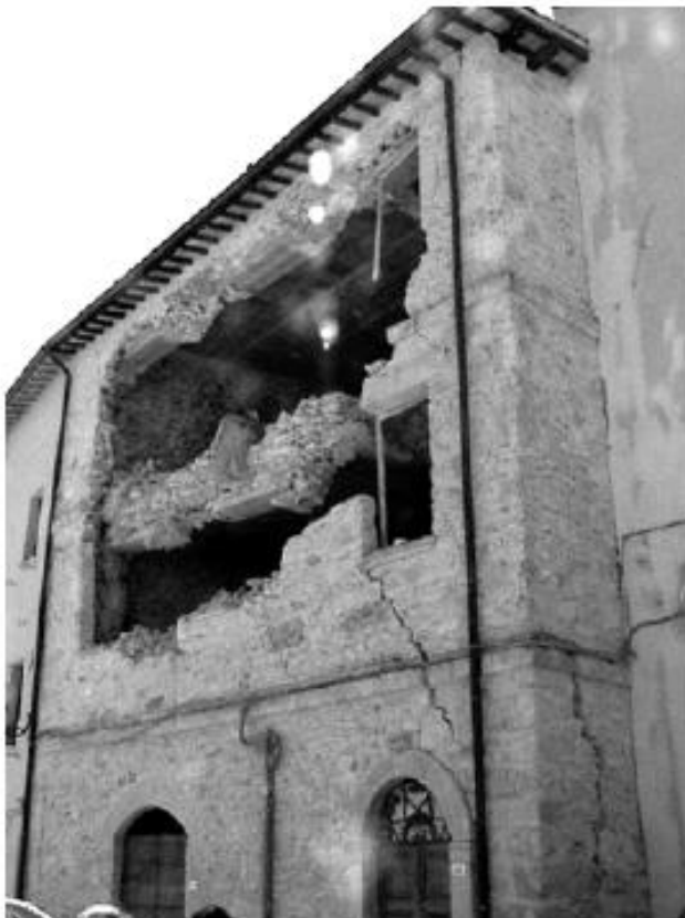
Figure 5.2.6.1 Damages after Umbria earthquake to a building repaired by introduction of concrete tie beams.
