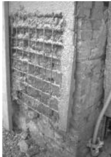
Fig. 6.1.5 Lack of connectors
