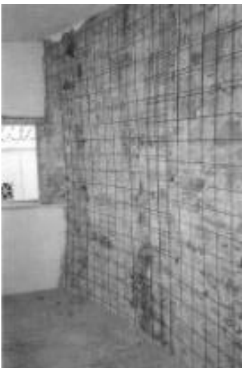
Figure 6.1.4 Lack connection Between the nets
