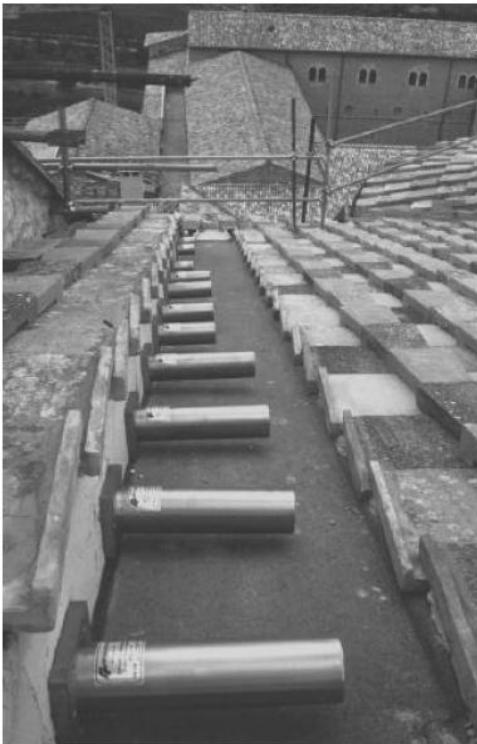
Figure 5.3.5.2 Shape memory alloy devices installed in the Basilica of San Francesco in Assisi.
