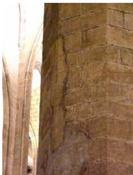
Figure 2.39– Splitting of material in pier
