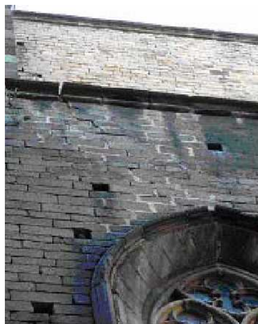
Figure 2.30 – Inclined crack from window towards tower
