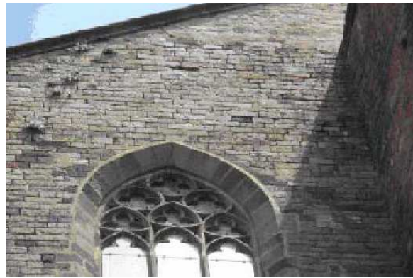
Figure 2.32 – Vertical crack in the upper wall of façade
