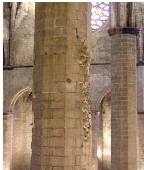
Figure 2.19 – Current view of the third pier at left side, damaged due to 1936 fire
