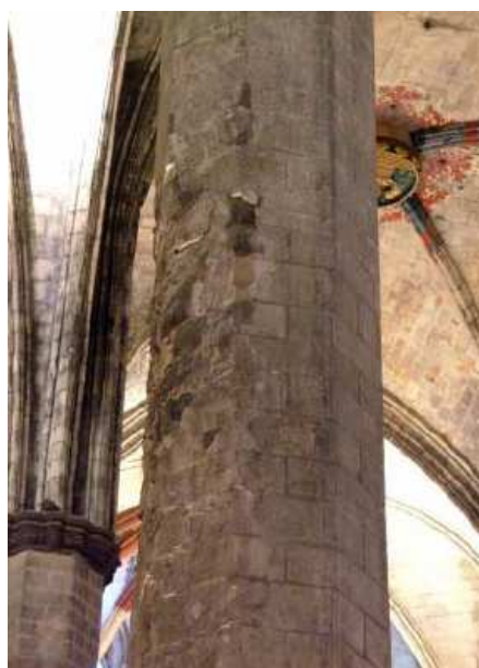
Figure 2.38 – Loss of material in pier 3 West
