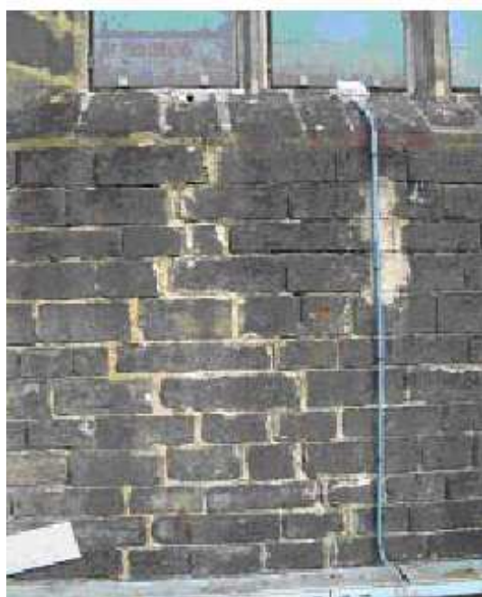
Figure 2.29 – Vertical crack below window
