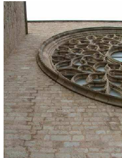
Figure 2.34 – cracks near rose window
