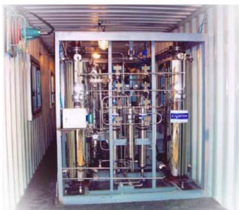
Hydrogen Generating System by Water Electrolysis in a container
