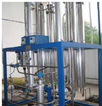
Hydrogen Generating System Purifier
