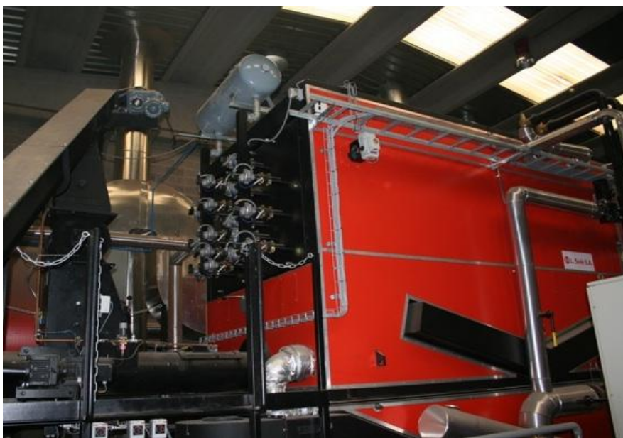
FIGURE 34. Biomass boiler, Molins de Rei biomass plant. Source: L.Solé
