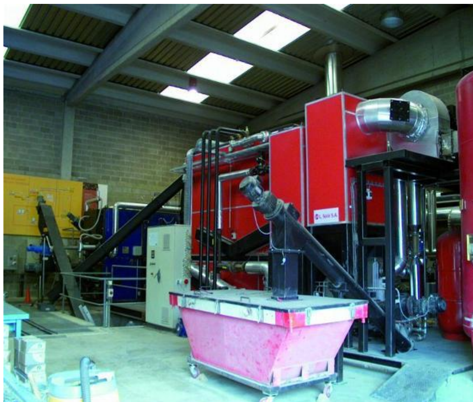
FIGURE 35. Biomass boiler, Molins de Rei biomass plant. Source: L.Solé
