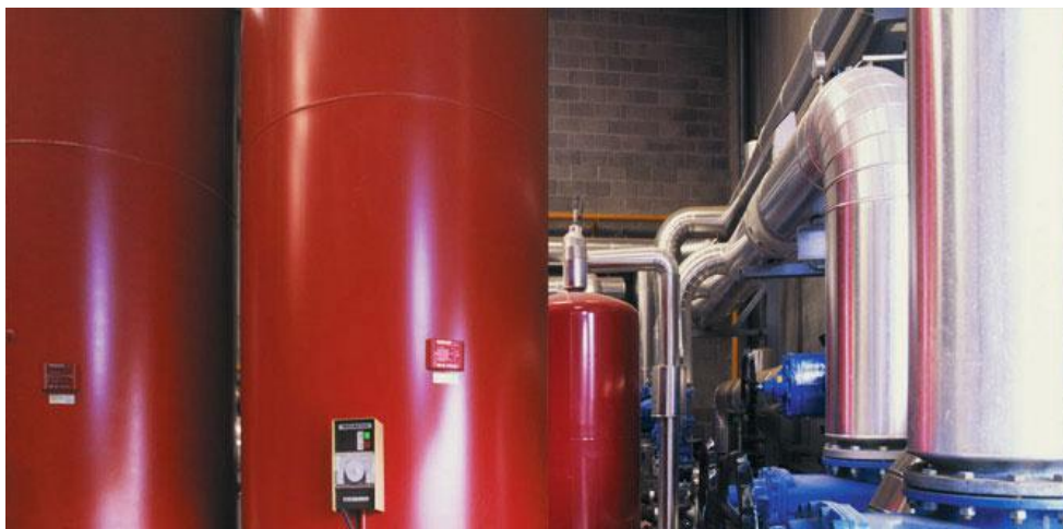
FIGURE 30. Molins de Rei biomass plant. Hot water production & distribution network. Source: L.Solé.
