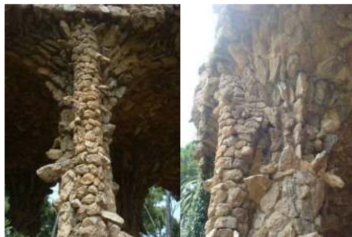
Figure 3.15 Stem-like columns in the north side of the bridge of the lower viaduct
