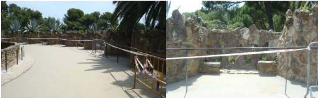
Figure 3.18 Left: View of the deck of the bridge Right: Detail of the bench at the south side of the deck of the bridge at its current state with forbidden access due its instability problems
