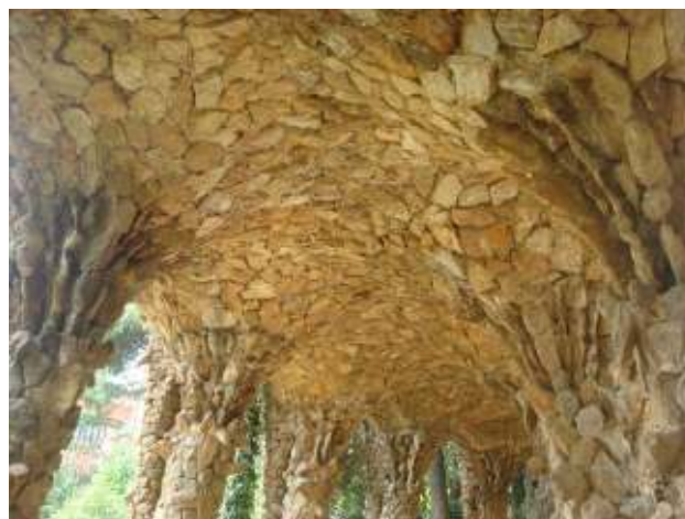
Figure 3.17 The fan vaulting of the lower viaduct. The transmission of the load is done through the capitals that have a mushroom shape.
