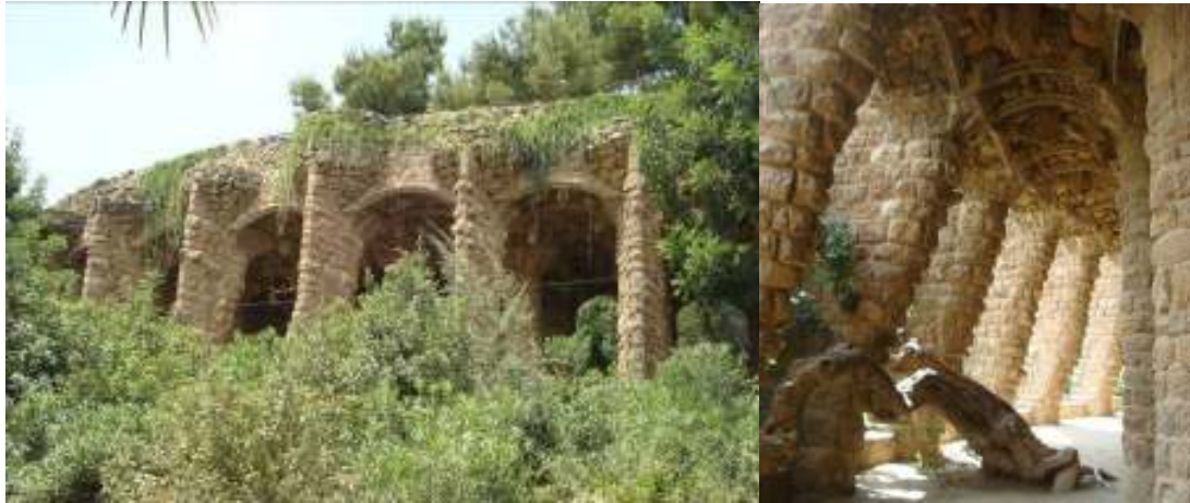
Figure 3.6 Left: View of the middle viaduct Right: Bearing structure of the middle viaduct
