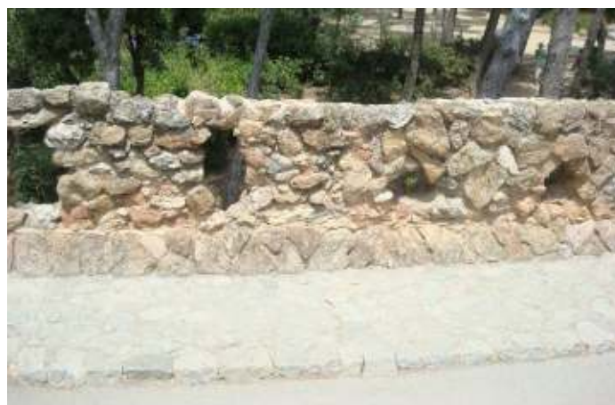
Figure 3.20 Railing at the north side of the deck of the bridge of the lower viaduct
