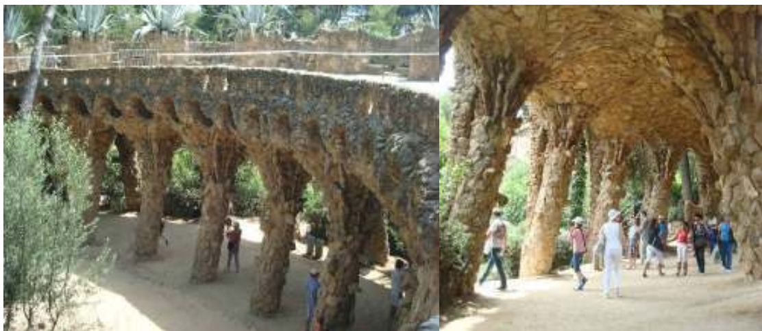
Figure 3.5 Left: View of the lower viaduct Right: Bearing structure of the lower viaduct
