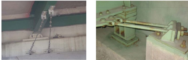
Figure E.3 Restrainer Cables (Left) and Restrainer Bars (Right) (Timothy et al., 2011)
