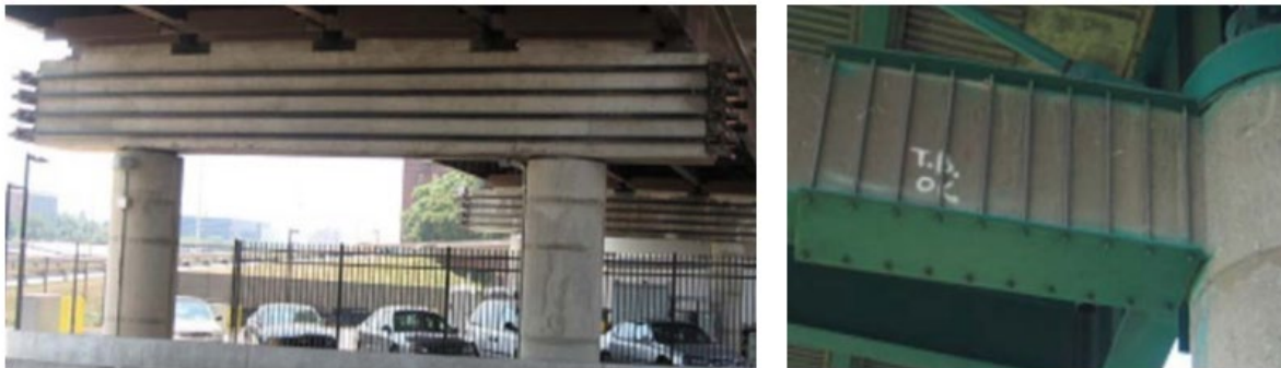
Figure 5 External Post-Tensioning (Left) and Shear Reinforcement (Right) for Bent Cap Strengthening (Timothy et al., 2011)
