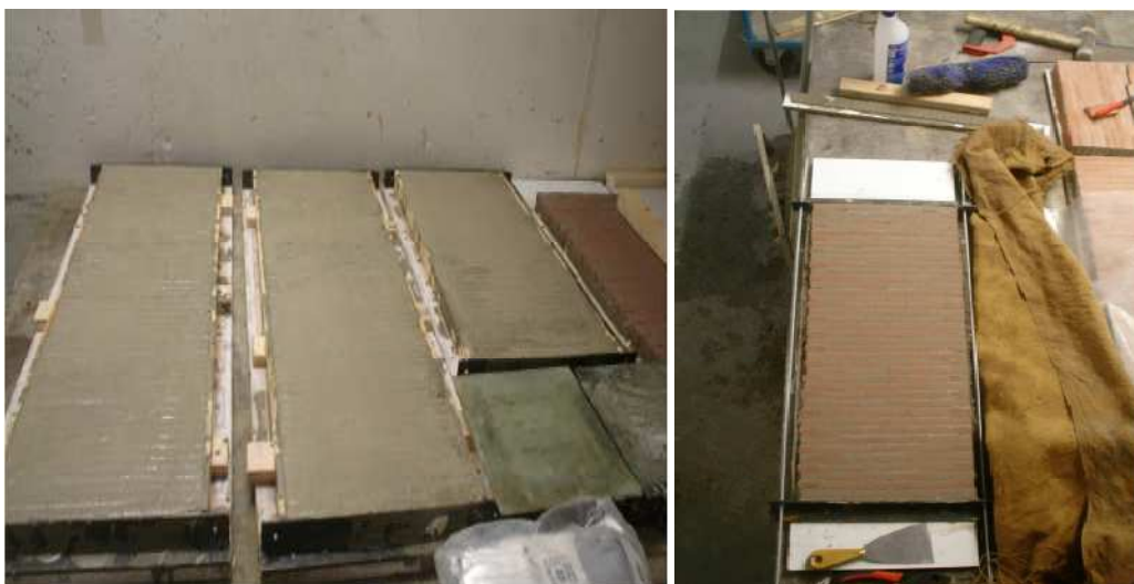
Figure 41: Wall after pouring of mortar (left) and wall after cleaning its surface (right).
