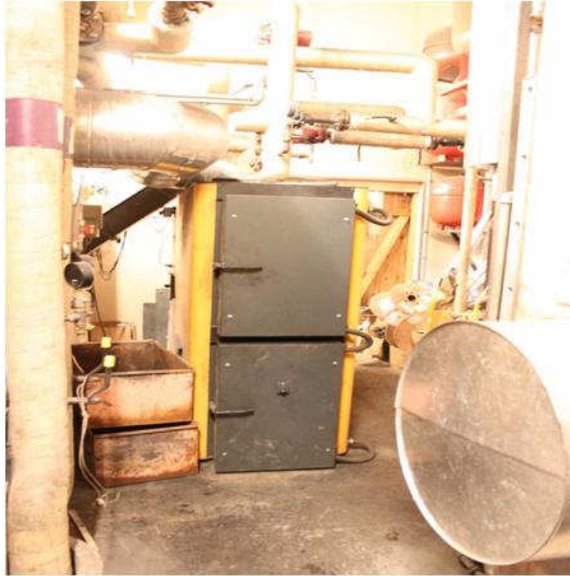
Picture 4.4.1: The first boiler was a granules Boiler (180kW)
