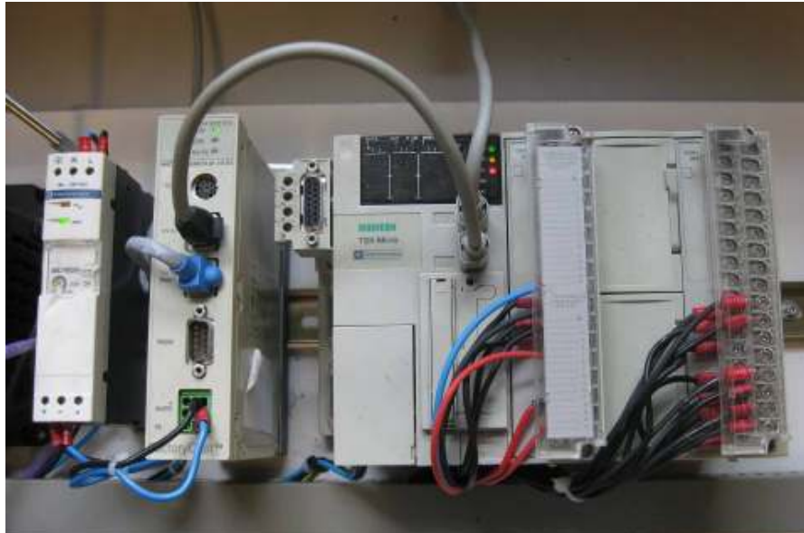
Figure 5.3. Power supply, TSX ETZ 410, TSX Micro 3722
