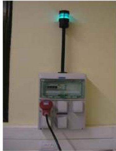
Figure 5.1. Main power supply
